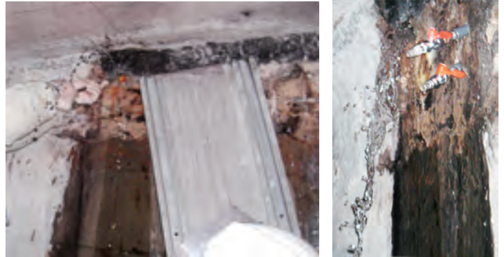
More than 20 liters of water is leaking from this area every minute.
