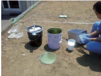
Preparation for construction. SKY-RGH diluted 10 times with water. Depending on the dilution ratio, drying time and hardness during drying change.
